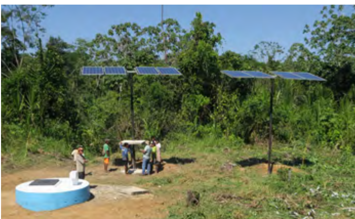
Shirintiari: the 8 solar panels near the well
