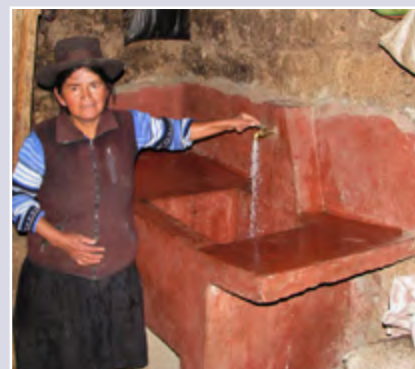
145 sinks were built in Huancapuquio, Pillucho and Huayracasca. This one was installed inside the house
