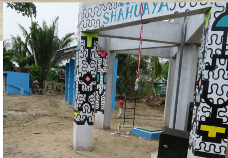
The columns of the reservoir painted with motifs and colors from the Shipibo-Konibo culture.
